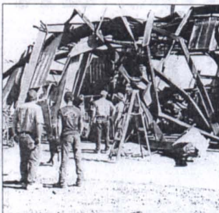
Special to The Commercial Farmers survey a twisted farm structure on Tarkington Road near the rice center.
